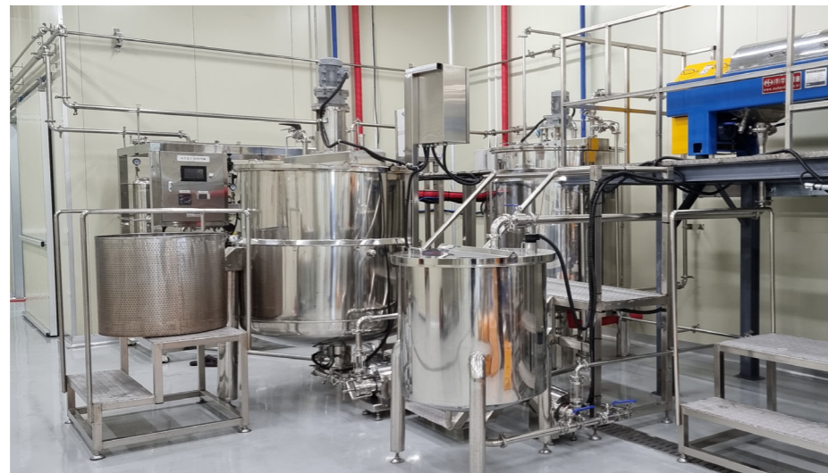
Auxiliary Storage Tanks Storage tanks for breaking down materials into enzymes and storage tanks for screw decanter centrifuge refined drinks. Equipment Auxiliary Storage Tank.
